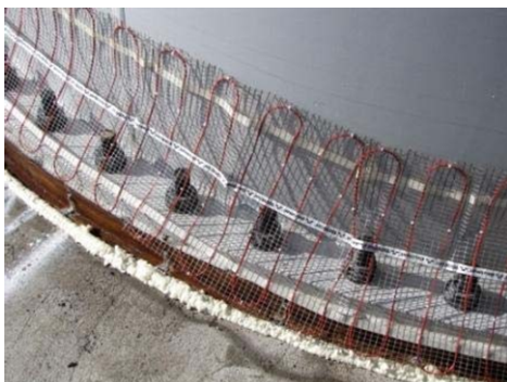
Heating elements to ensure minimum temperature
